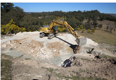
Work continues in order to build up and restore natural slope of the land.
